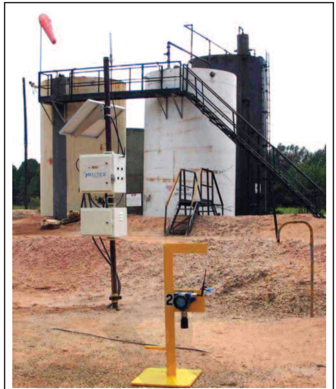
By installing monitoring systems on its pipelines, tanks, compressors and other equipment, Tellus Operating Group has reduced the amount of time its technicians spend going to and checking gauges. The company says the monitors enable it to respond to problems or warning signs before they lead to downtime.
